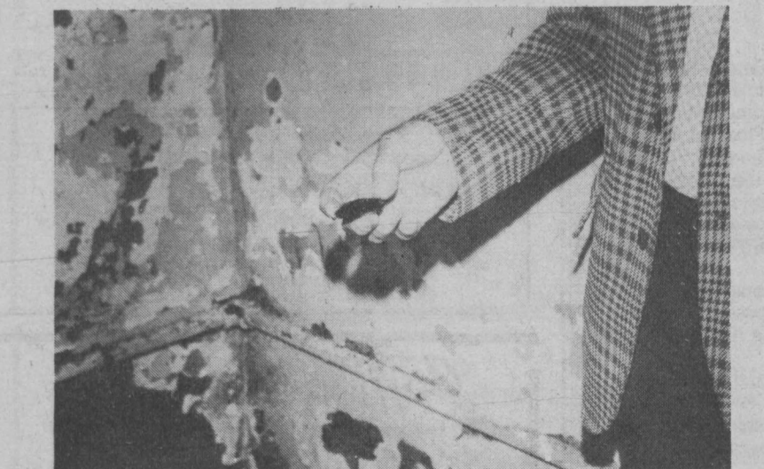
Charles Elyer holds a piece of tar which blocked the drains at the Community Center, causing damage.
