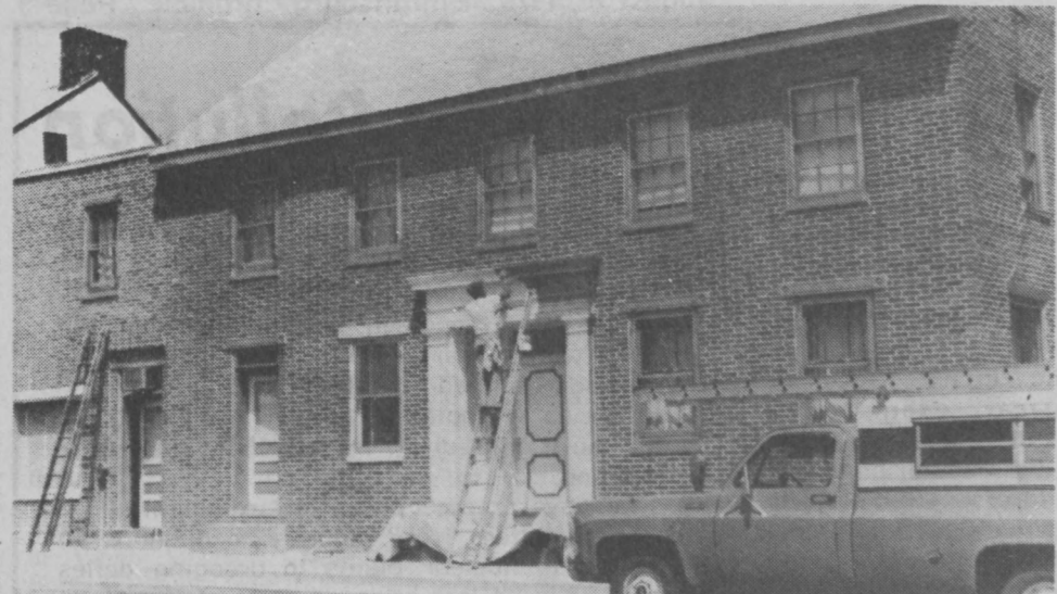
Bill Stultz puts the finishing touches on the recently sandblasted Adams House on West Main St. (Photo by Becky Brown)
