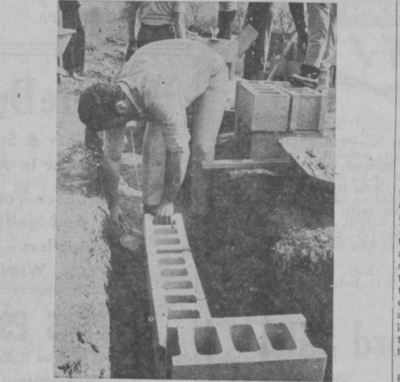
Joseph Topper had a chance to practice some of the skills he had learned in class as construction got under way.
