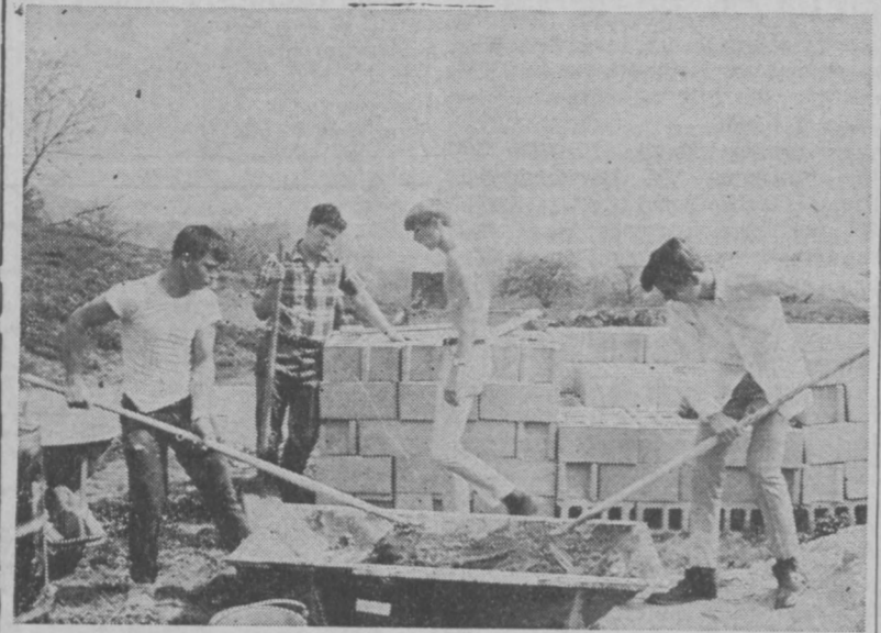
Jerry Ridenour, Frank Adams, Gary Dingle and David Fogle (l-r) are shown during the construction
