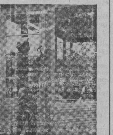
During construction, carpenter nails one of ponderosa pine combination doors in place between 4x4 posts supporting roof.
