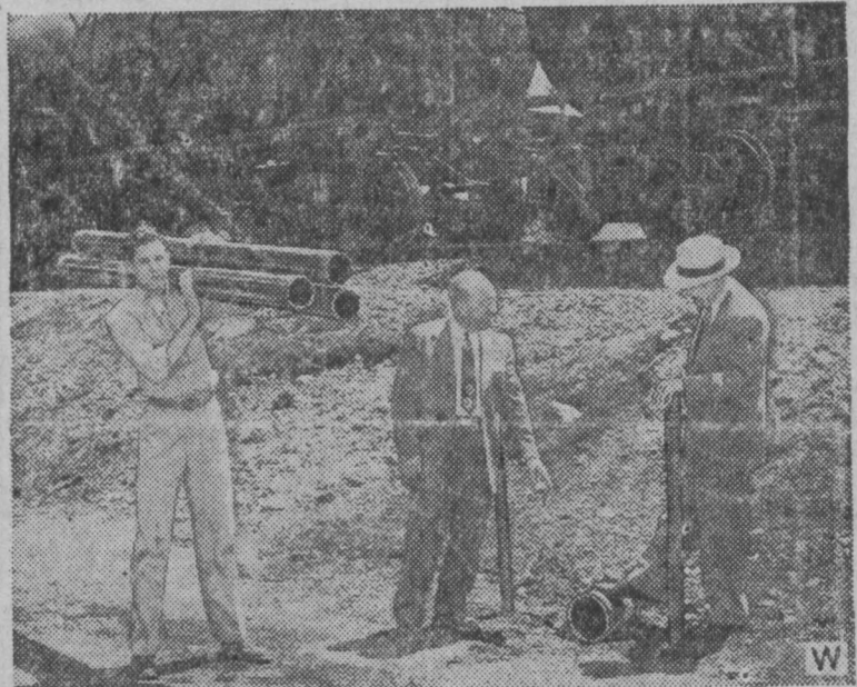
At least twice a day for the past three years a 128-ton switch engine has pulled loaded tank cars, at 20 tons each, over a culvert installation of eight-inch Orangeburg pipe, graphically demonstrating the strength of light-weight Orangeburg Manufacturing Company bituminized-fibre drain and sewer pipe. Company officials make periodic inspections. Despite the terrific pressure the pipe remains in perfect condition.
