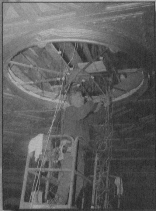
Bill Rigby, an electrician with Hull's Electric, Gettysburg, PA, works on the wiring installation for a huge light fixture that will be installed to replace the antique unit that once hung there. The original lighting was removed during a previous remodeling and the antique chandelier stored at the Gettysburg College, but has since been lost. The new stained glass chandeliers were specially designed in the style of the original. Photo by Dick Bloom / The Dispatch.
