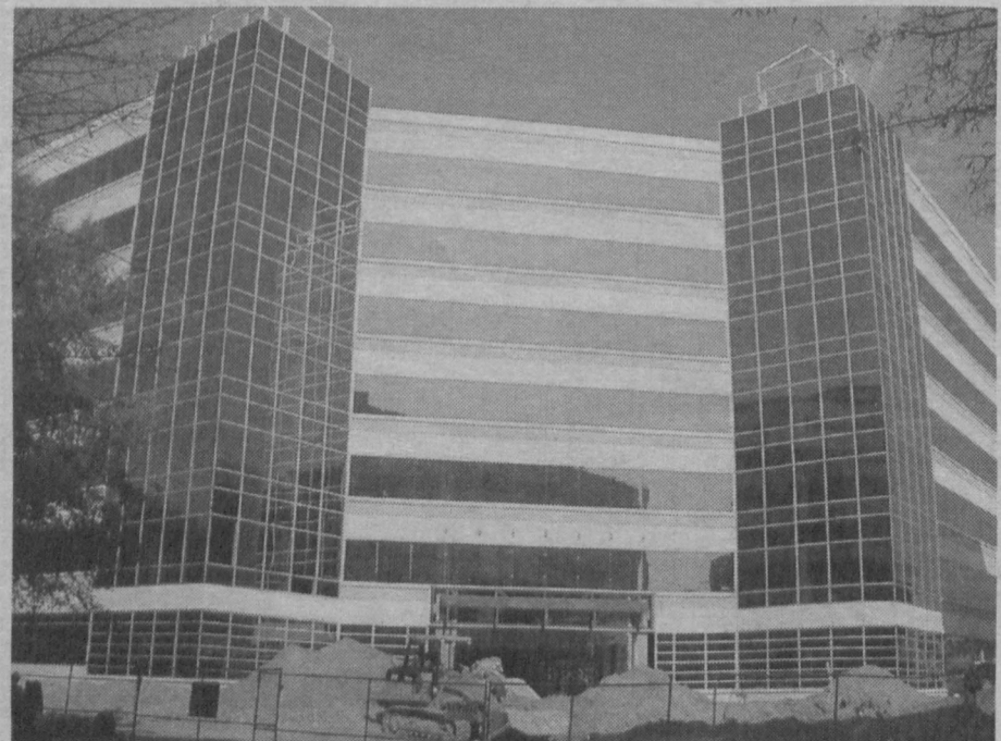
Willow Oaks, a seven-floor office building in Fairfax, Va., in the final stages of glass installation.
