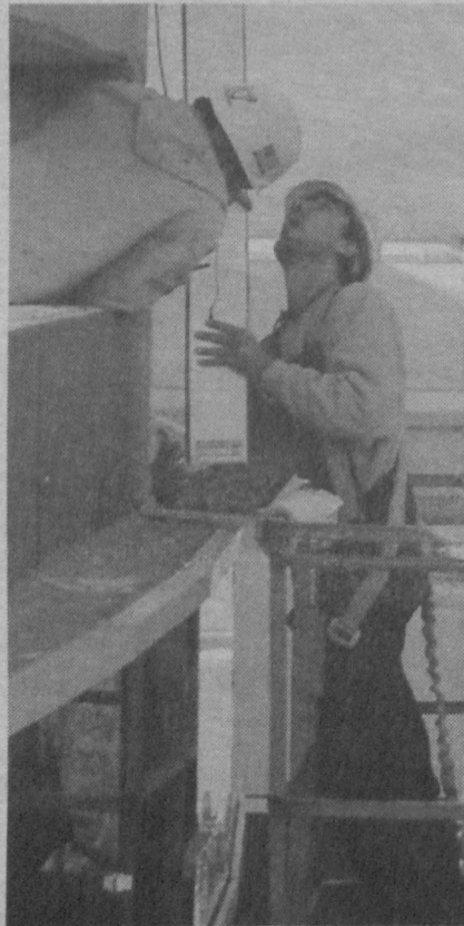
Company foreman Kevin Horan, a.k.a. "Red Dog," left, and Wayne Kauffman, company glazier, erect framework on the 7th floor of Willow Oaks high rise.
