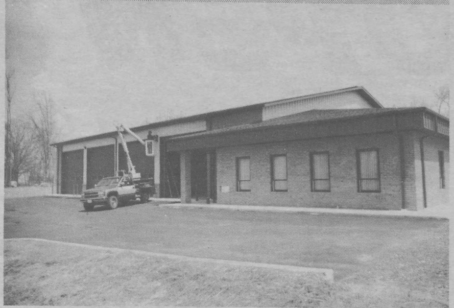
Finishing touches are being applied to the new Rocky Ridge Engine House on Motter's Station Road.
