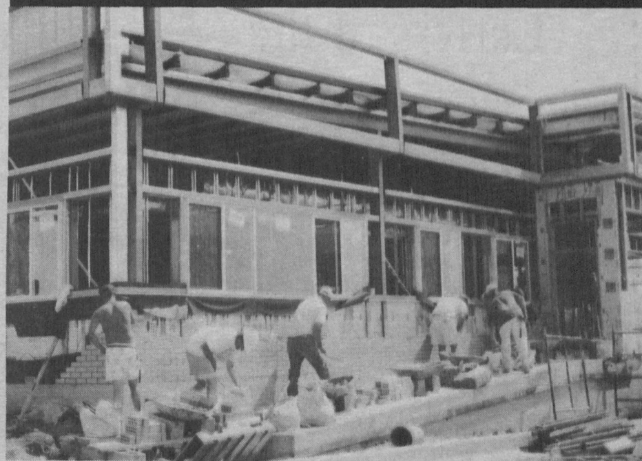
Construction moves along at a rapid clip on the new Up-County Family Center on East Lincoln Avenue. A Dispatch Photo
