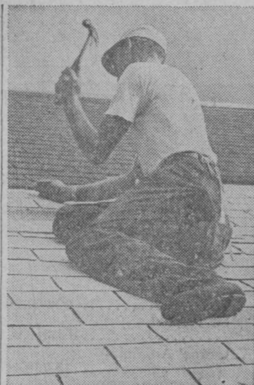
Roofer applies new roof of asphalt shingles directly over old roof, saving mess and expense of ripping off old material.
