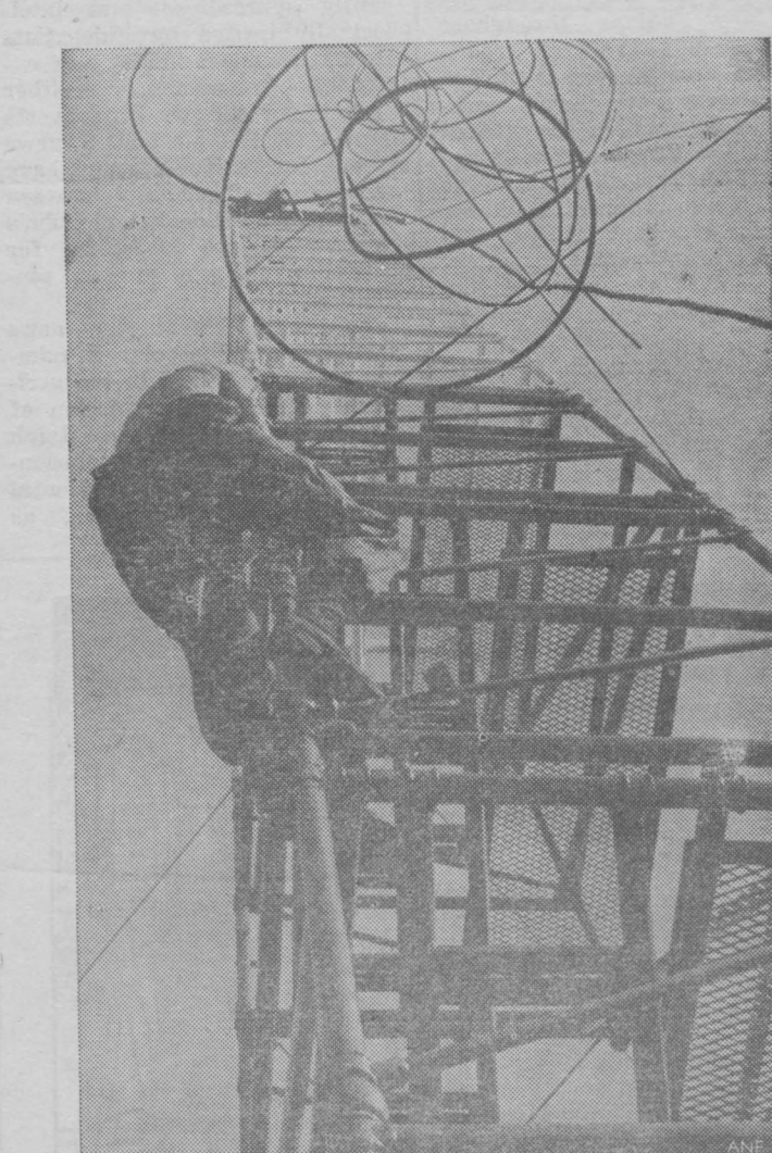
WIRED FOR SOUND—A tangled maze of wire poses a temporary problem for Sgt. Lonnie C. Baldwin while working on the construction of a radio tower in the Republic of Vietnam. Sergeant Baldwin, of Rowe, Va., is a member of the 327th Signal Battalion, 1st Cavalry Division (Airmobile). (U.S. Army Photo by Pfc James McCabe)
