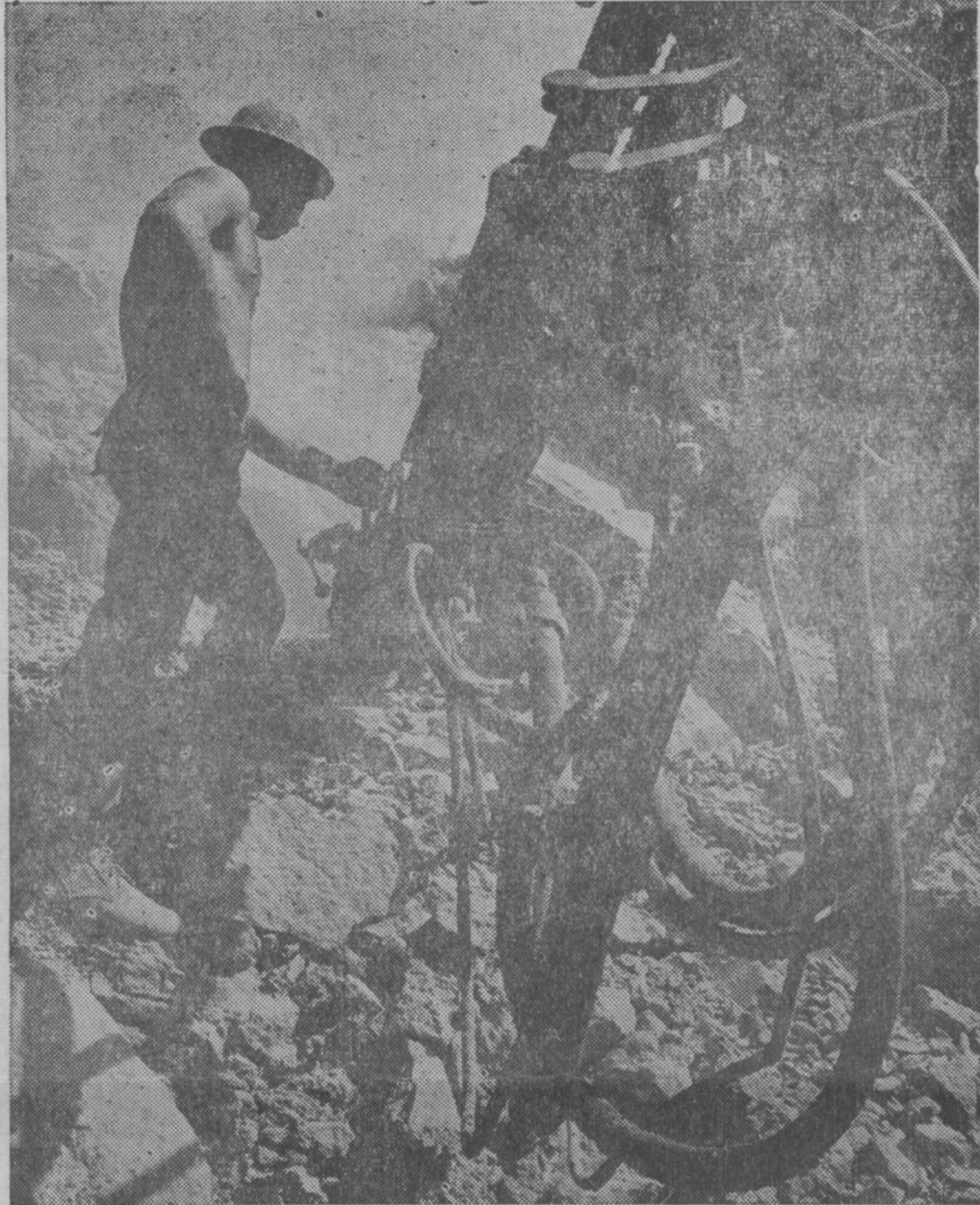
With an air drill, a soldier of the 79th Engineer Group sinks a hole for explosives in a rock quarry near Tay Ninh, Vietnam.
