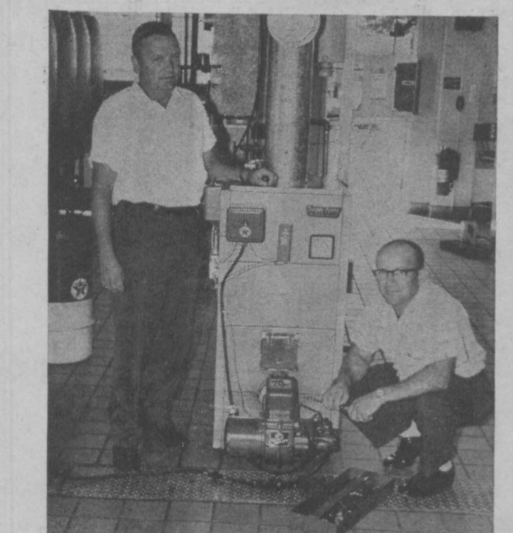
JET-AGE HEATING EXPERTS—Charles F. Stouter (l), Texaco Distributor, and Charles Hartdagen, service manager, Emmitsburg, Md., are recent graduates of the Advanced Service and Installation School on Oil Heating Equipment held at the Texaco Research Center, Beacon, N. Y. They are shown in the new heating oil laboratory with test equipment during classes for Texaco Fuel Chief marketers and their service managers. Graduates undergo intensive training in the latest techniques and developments of all phases of modern domestic oil heating.
