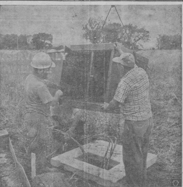
Weighing only 666 pounds and 28 1/2-inches high, an Allis-Chalmers transformer installed in a Janesville, Wis., subdivision is easily maneuvered into place on its concrete pad. The subdivision is the first in the state with both electrical and telephone wires buried together in a common trench. Allis-Chalmers acted as general contractor for the entire project.
