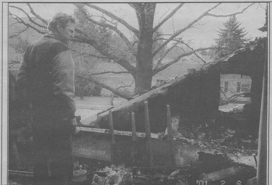
Dr. Robert Henke surveys the damage done to his home by an electrical fire. Photo courtesy Dolores Henke
