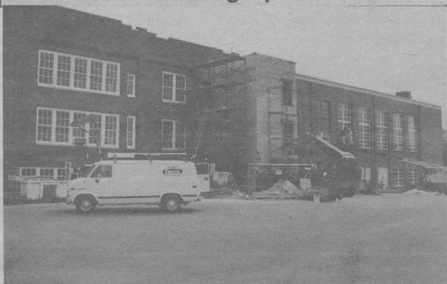
The old school "ain't what she used to be." As the present-day Emmitsburg Community Center, the building is undergoing modifications to comply with ADA regulations. A new elevator shaft rises in the area of the new main entrance to the building.
